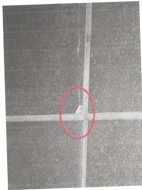
Figure 3.9 : Bathroom 'Chipping' defect
