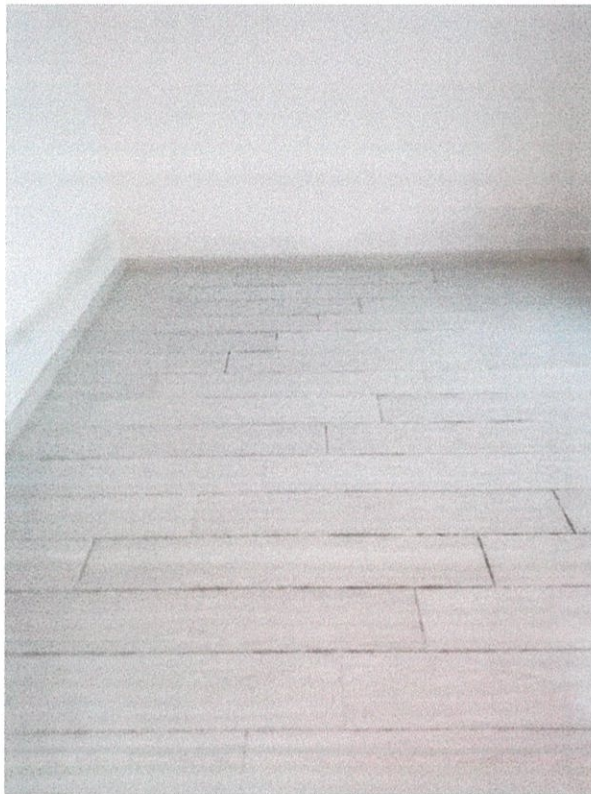
Figure 3. 15 : Laminated Parquet floor defect
