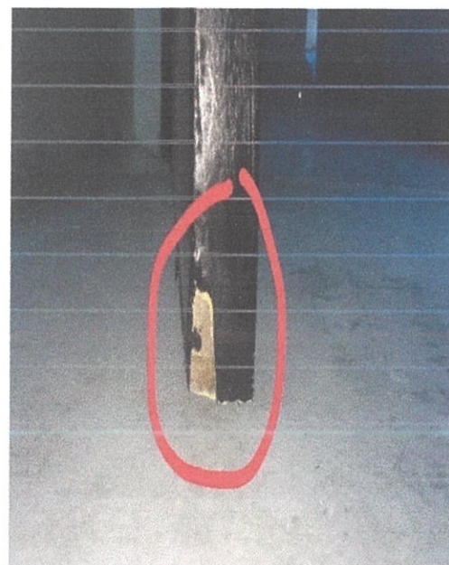
Figure 3.23 : 'Door leaf' defect
