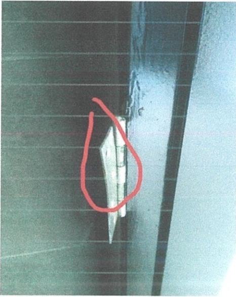
Figure 3.20 : Door frame 'Hinge' defect
