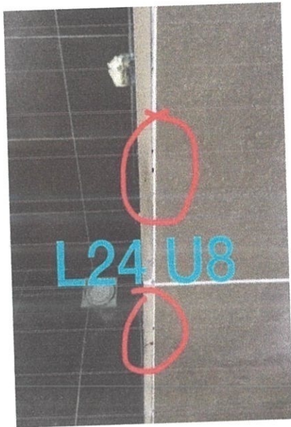
Figure 3.8 : Bathroom 'Grouting' defect
