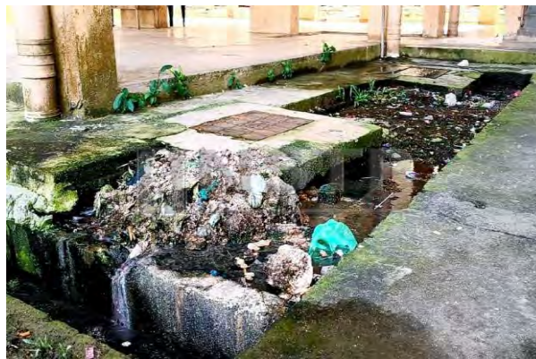
Figure 2 : Failure at almost all of the sewer system at PPR Taman Mesra, Sandakan Source: (Sidom, 2019)
