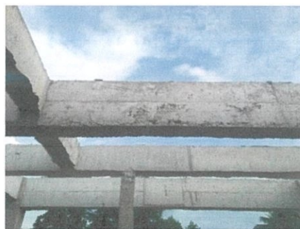
Figure 3.2.18: honeycomb at beam
