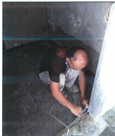
Figure 3.14: The tile layer covers the floor tiles for protection during tiling wall.
