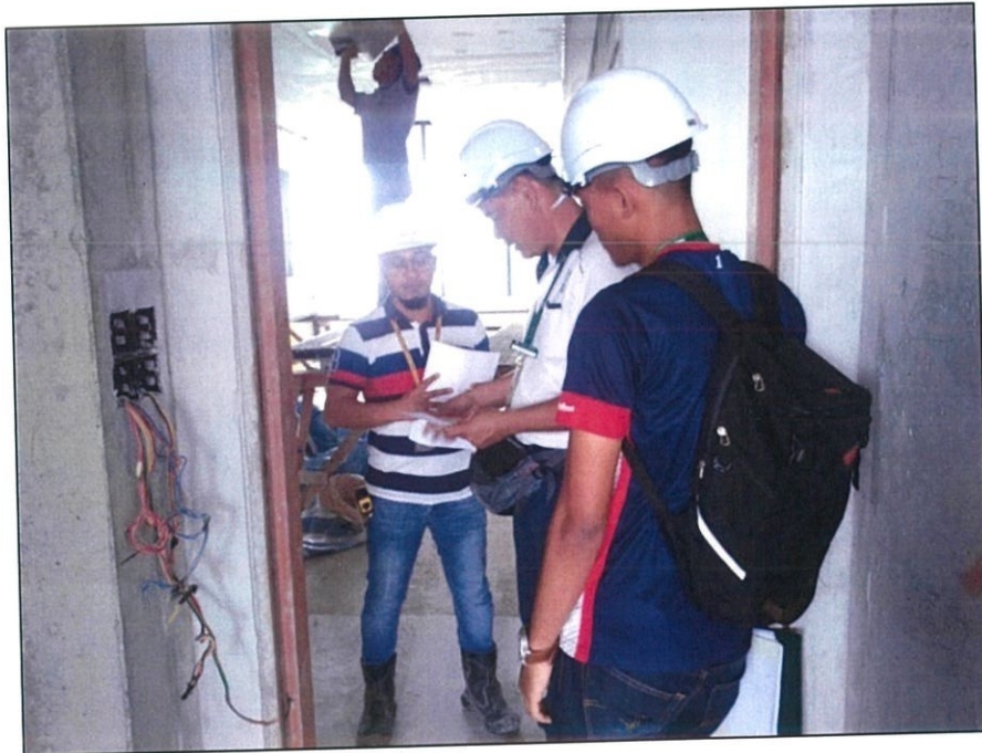
Figure 1.4: Discussion with site manager, site supervisor and client representative about the problem for install bathroom tiles.
