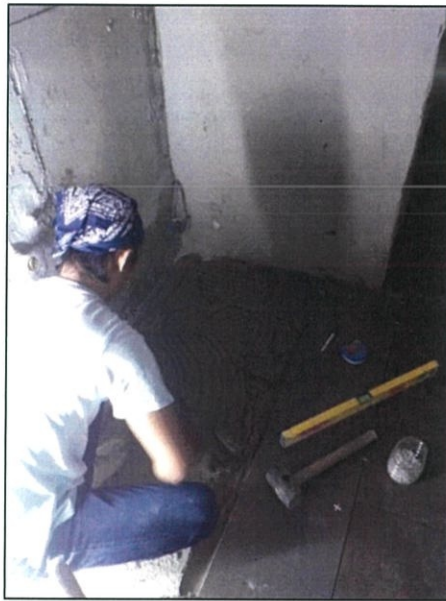
Figure 3.12: The tile layer continues install the floor tiles and put the 2mm spacer between it.
