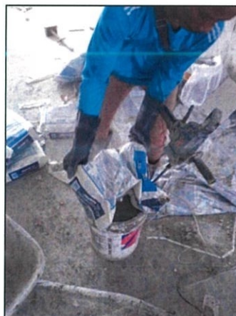
Figure 3.16: The tile layer preparing the Adesillex P9 cement for the adhesive of the wall
