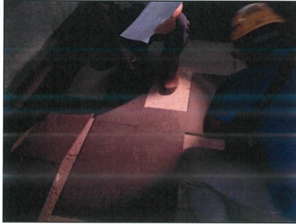
Figure 3.9: The tile layer laying out the tiles before start the installation process.
