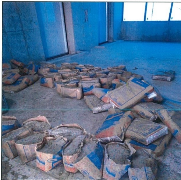
Figure 3.10: Preparation for mixing Kerabond T cement that use as adhesive for floor tiles.
