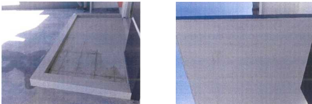
Figure 13 Dampness at car porch roof and balcony
