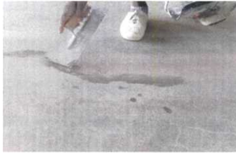
Figure 14 Method to rectified plastering crack at floor rendering
