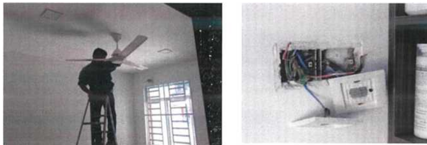
Figure 11 Defect at Azalea where the fan is not working and the problem of switch
