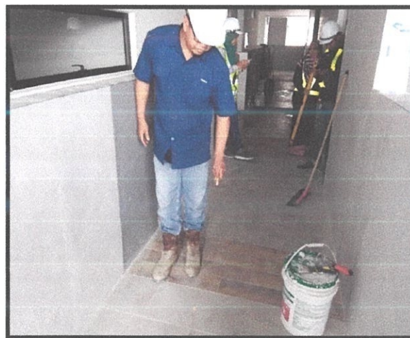
Figure 3.3.1(g) : Inspector of works (IOW) inspect PDI : hollowness of tiles at the corridor
