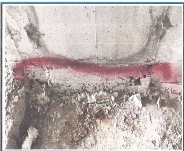
Figure 3.3.2(t) : Defects: honeycombs
