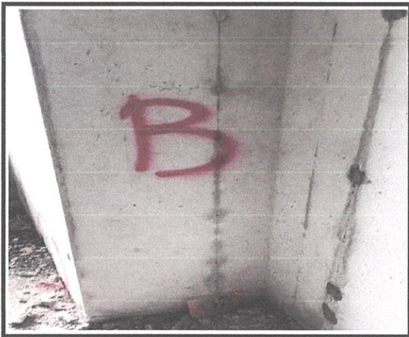
Figure 3.3.2(r) : Defects: bulging
