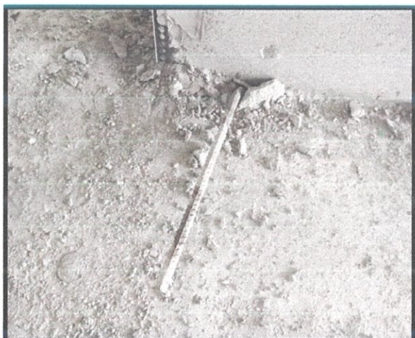
Figure 3.3.2(u) : Defects: steel exposed
