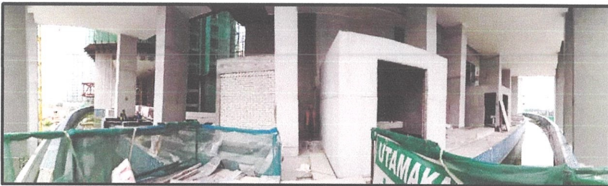
Figure 3.0.(e) : Panorama view of the progress from the infinity swimming pool area and the jacuzzi area
