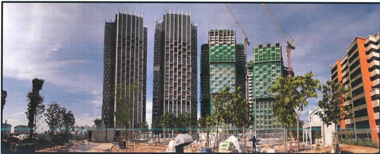
Figure 3.0.(b) : Panorama view of the progress from the landscape area above the carpark, from the left is Tower A1, then Tower B1, Tower A2 and Tower B2
