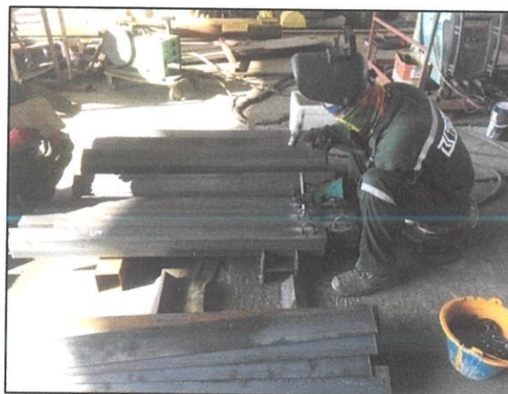
Photo 3.9: Round bar bracket are welded into the surface of the angle steel bar
