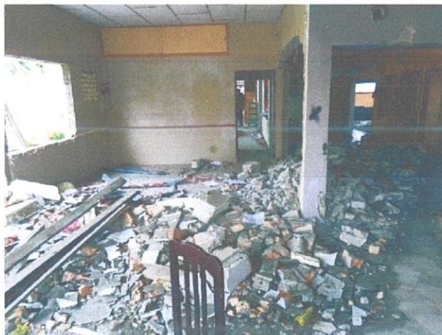
Figure 2.2.3 : Some broken wall
