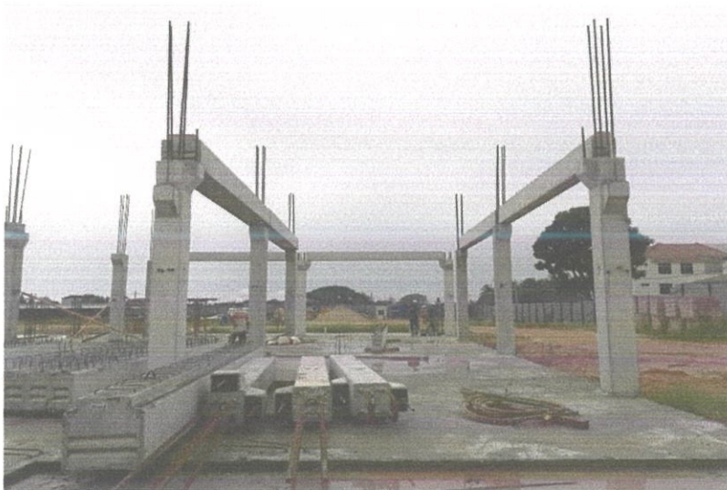
Photo 3.1: Industrial Building System been installed in Project Klinik Kesihatan (Jenis 3) Pauh, Perlis.
