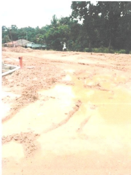
Figure 3.22: The water puddles on the ground
