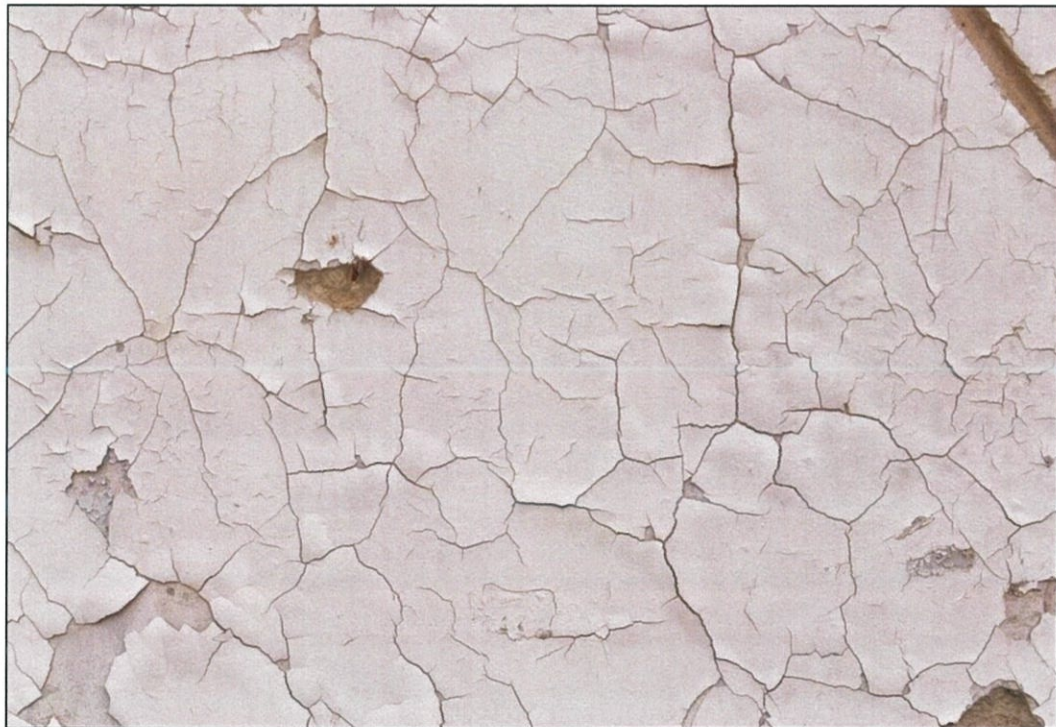
Figure 3.6: Defective Plaster Rendering
