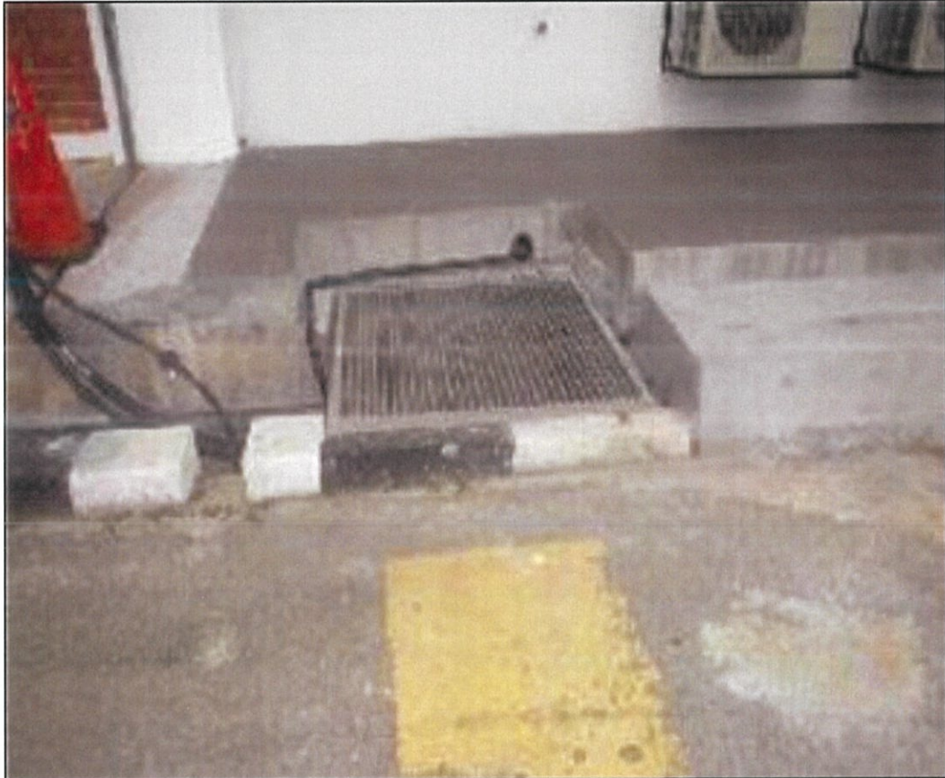
Figure 3.11: Exposed Electrical Cables
