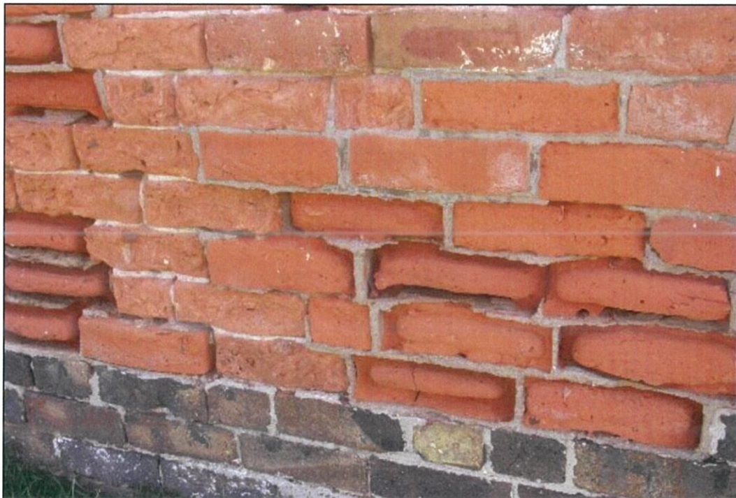
Figure 3.7: Erosion of Mortar
