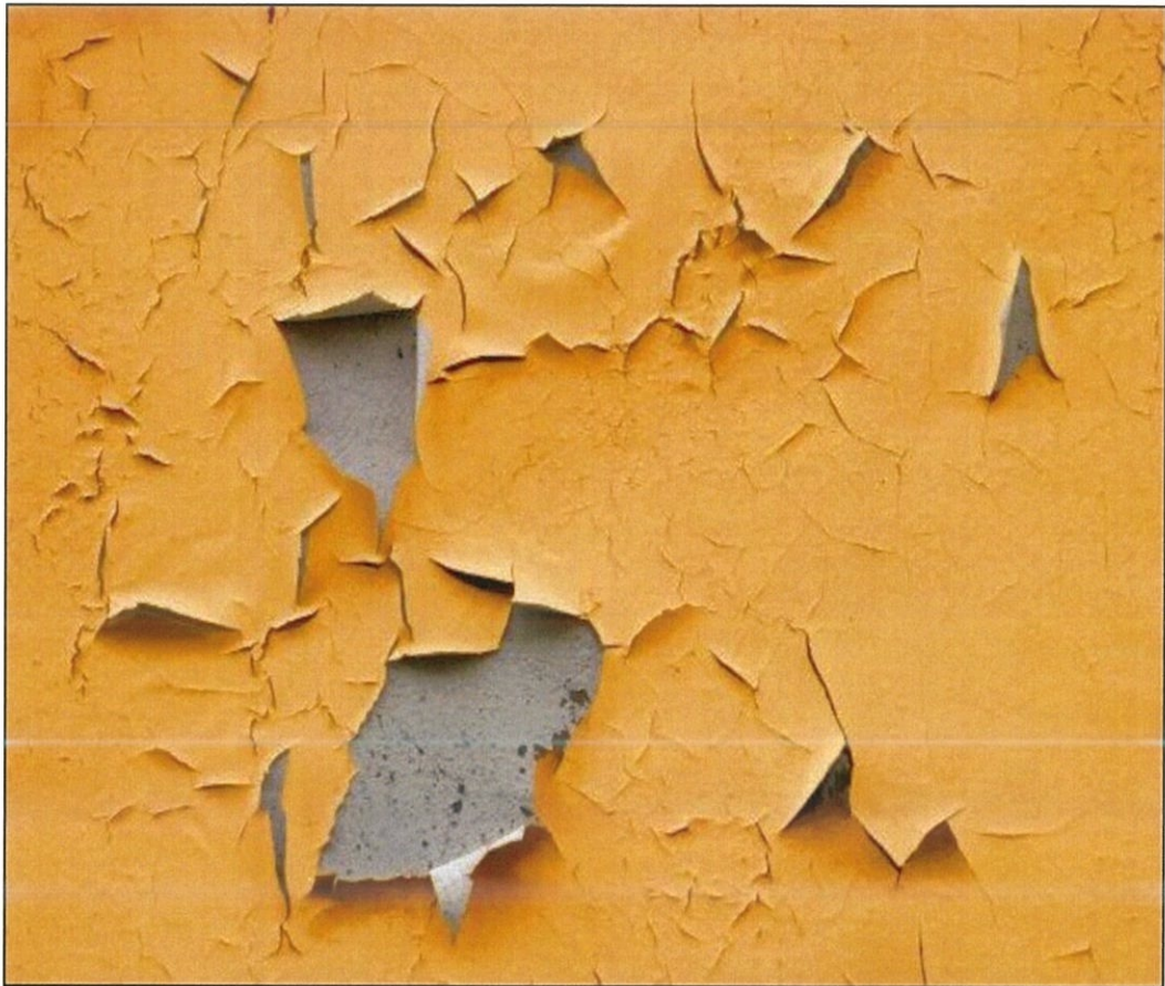
Figure 3.5: Peeling of Paint
