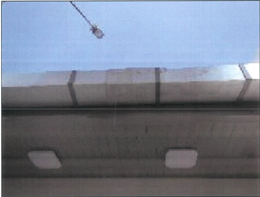
Figure 3.9: Gutter Brackets Rusty
