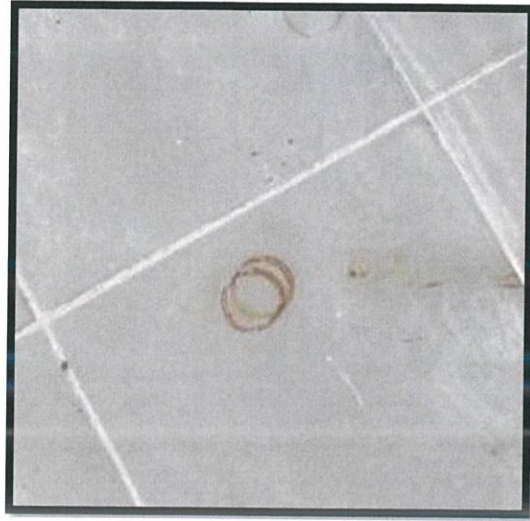
Figure 29 Stain on tiles
