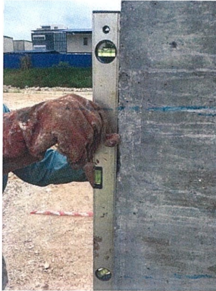
Photo 3.12: Spirit level are used to ensure the pile is in the straight position.
