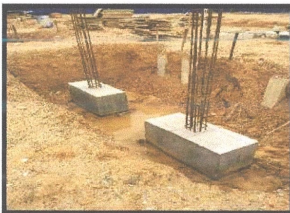
Photo 3.16: Condition of pile cap size 1300 mm x 550 mm after formwork was uninstalled.
