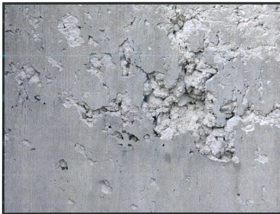
Figure 8: Honeycomb in Concrete. (Source: Civilengineernotes.com)
