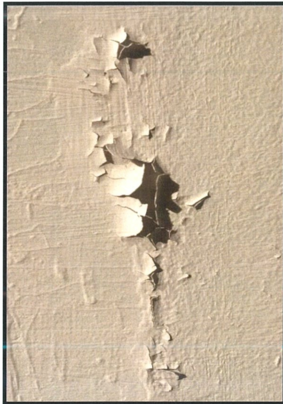
Figure 7: Peeling Paint in House Unit No. 20. (Source: Hijauan Damai Sdn. Bhd.)
