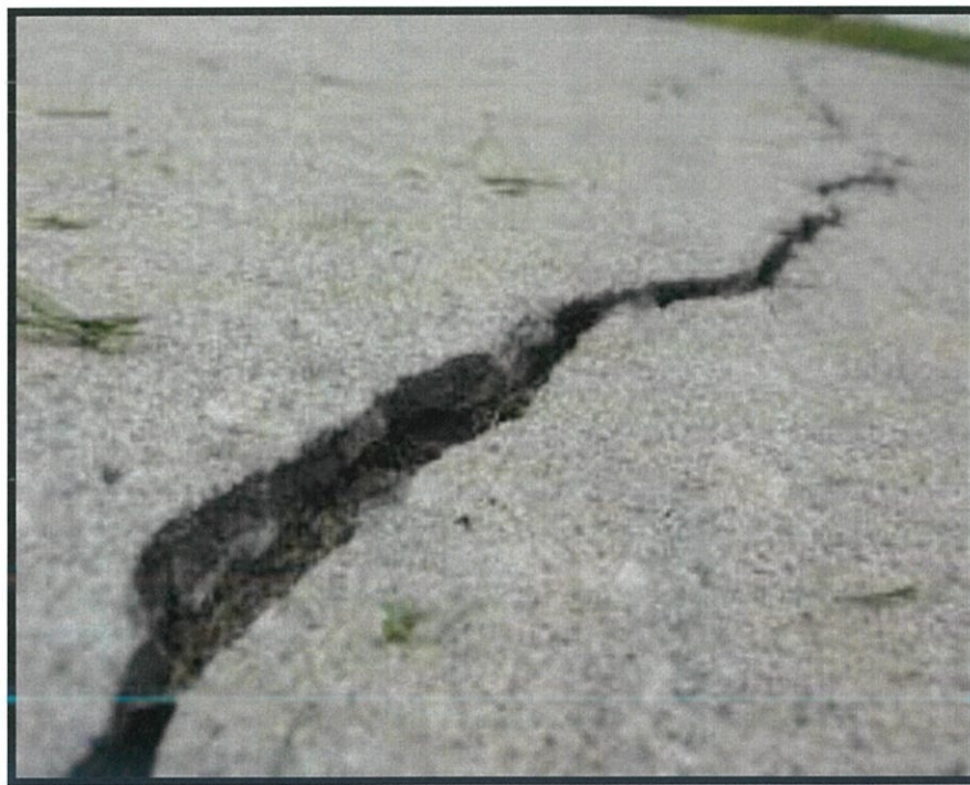
Figure 4: Settling Crack. (Source: Hijauan Damai Sdn. Bhd.)
