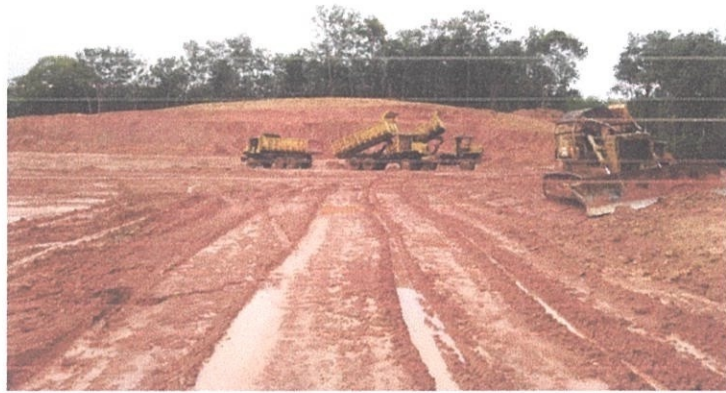
Figure 3.12 Machineries cannot being operate due to bad site condition
