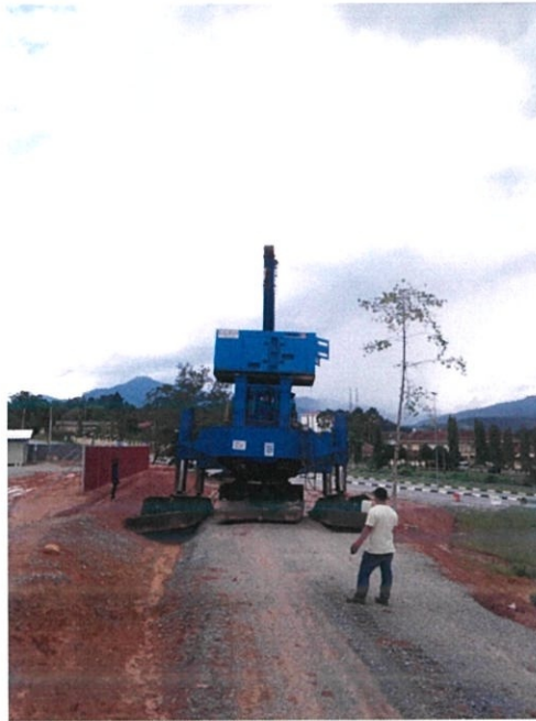
Figure 3.22 220kva generator placed on machine
