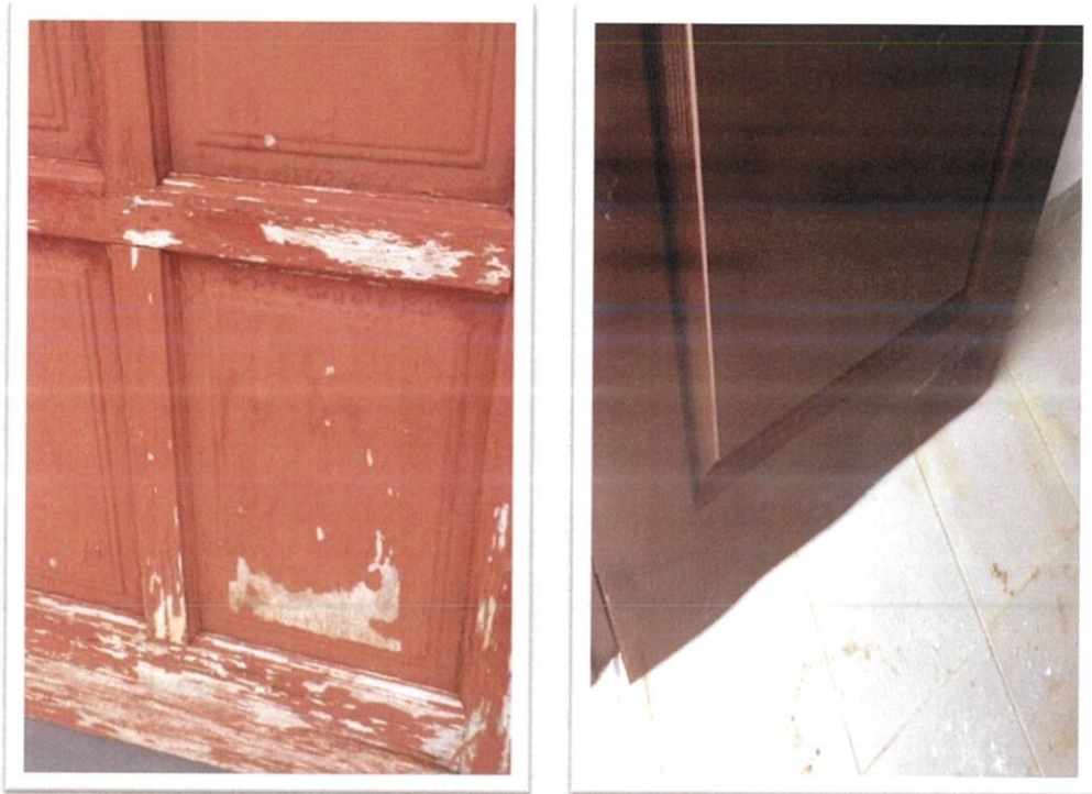
Figure 3.6 The front and back door condition due to deterioration
