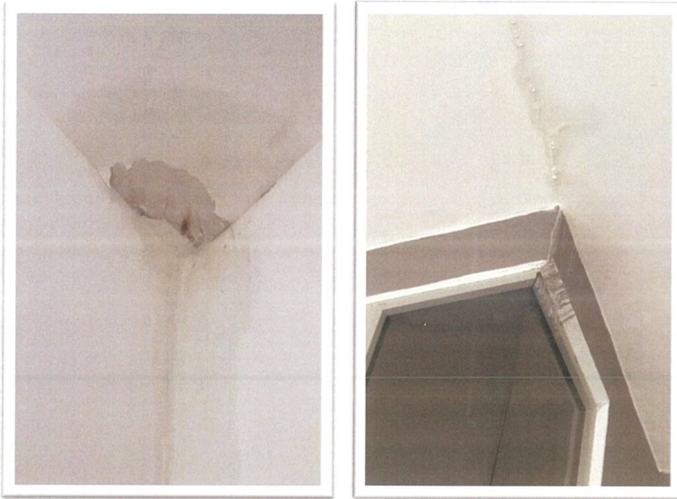
Figure 3.7 Water leakage condition
