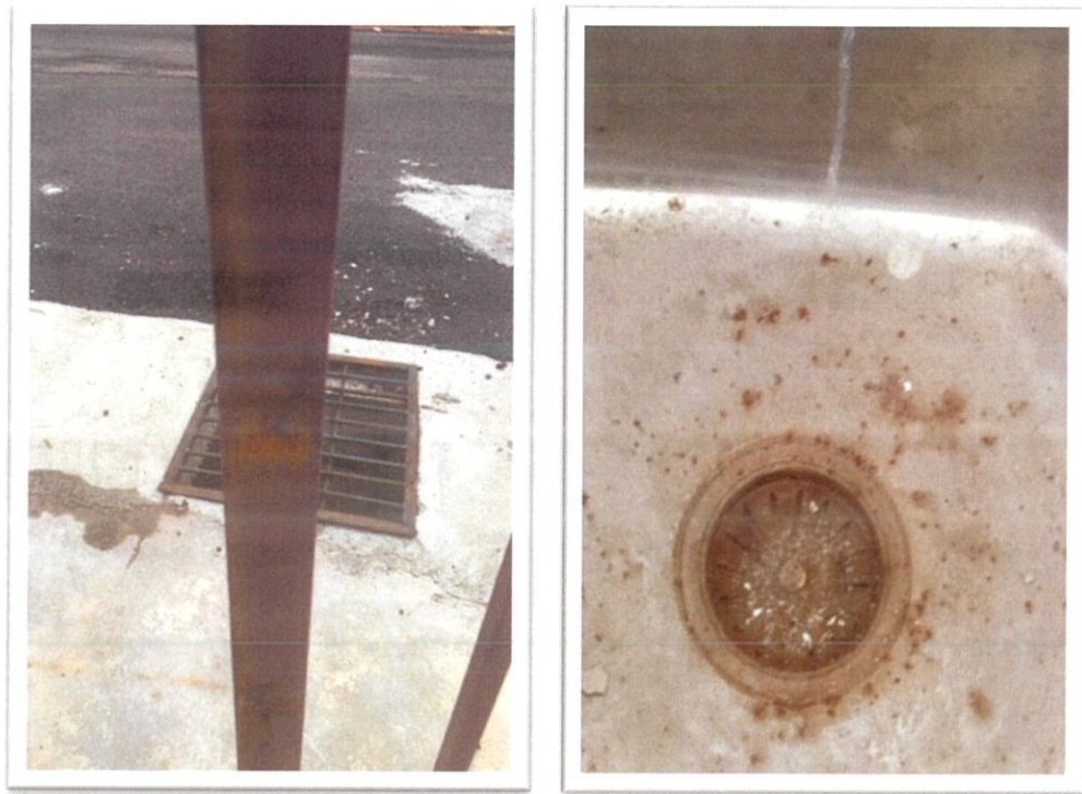
Figure 3.5 The affected gate and gasket by corrosion defect
