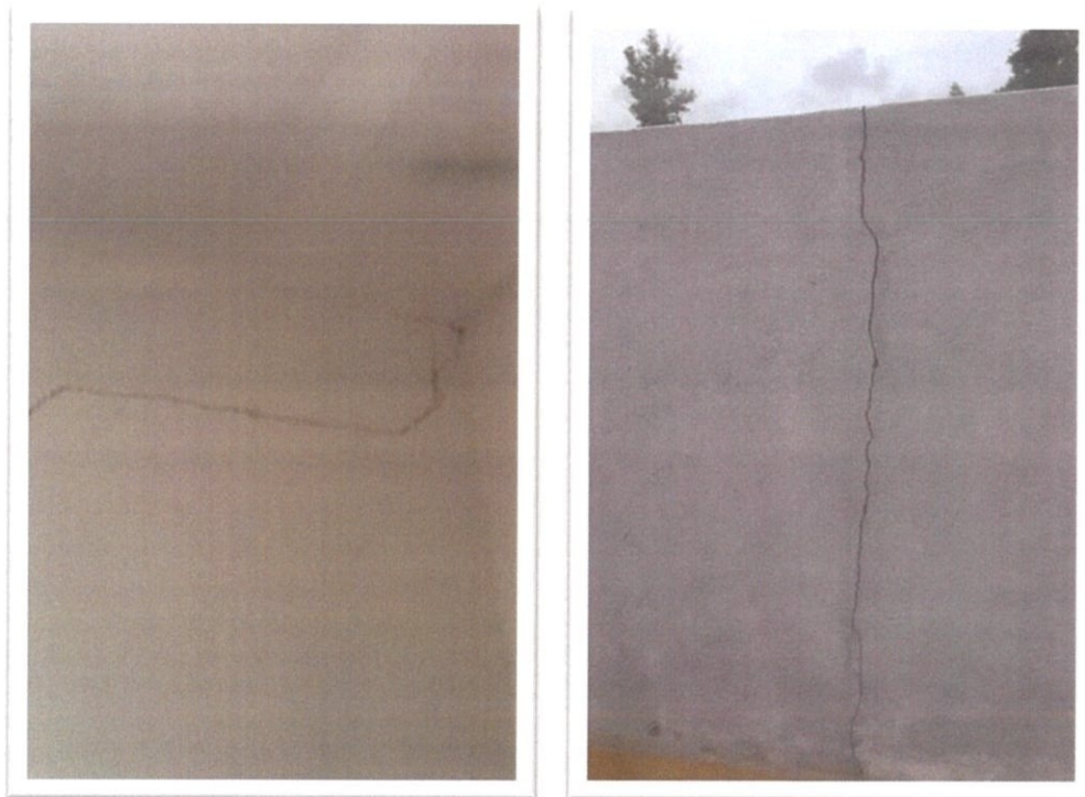
Figure 3.2 The example of cracking that can be found at Taman Salman
