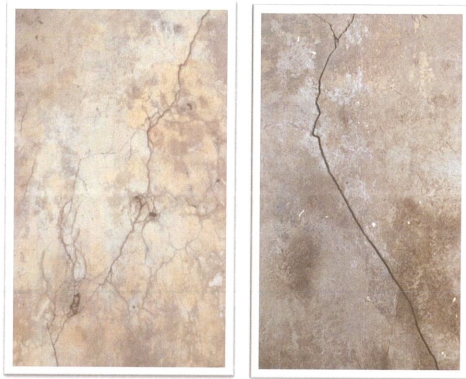
Figure 3.3 The form of cracking on the floor at the house porch
