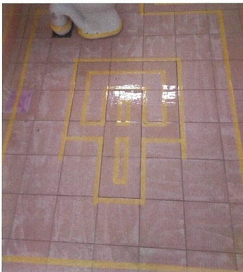
Figure 22 - The mixture apply on the floor for the first layer are done.
