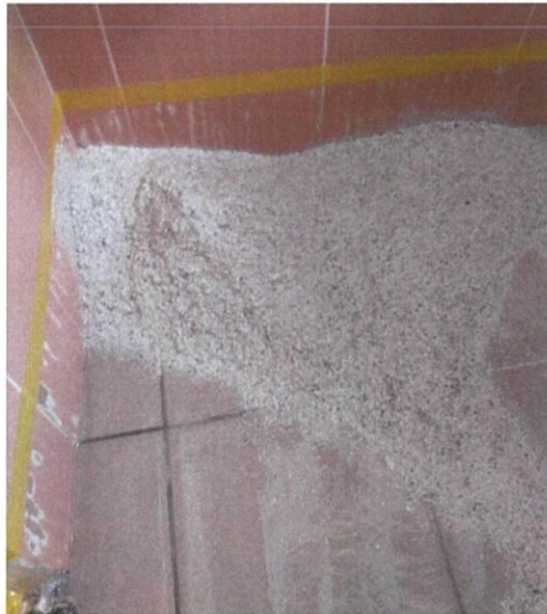
Figure 26 - White flakes for the skirting around the toilet.
