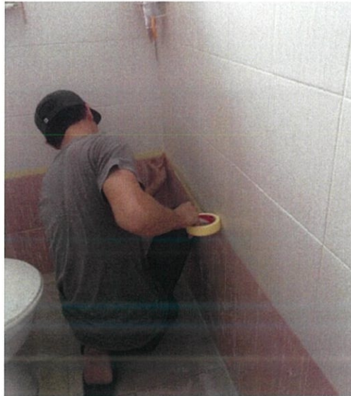
Figure 13 - tape around the toilet.
