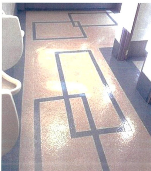
Figure 30 - Epoxy flooring. (Source: epoxyxpert.com)
