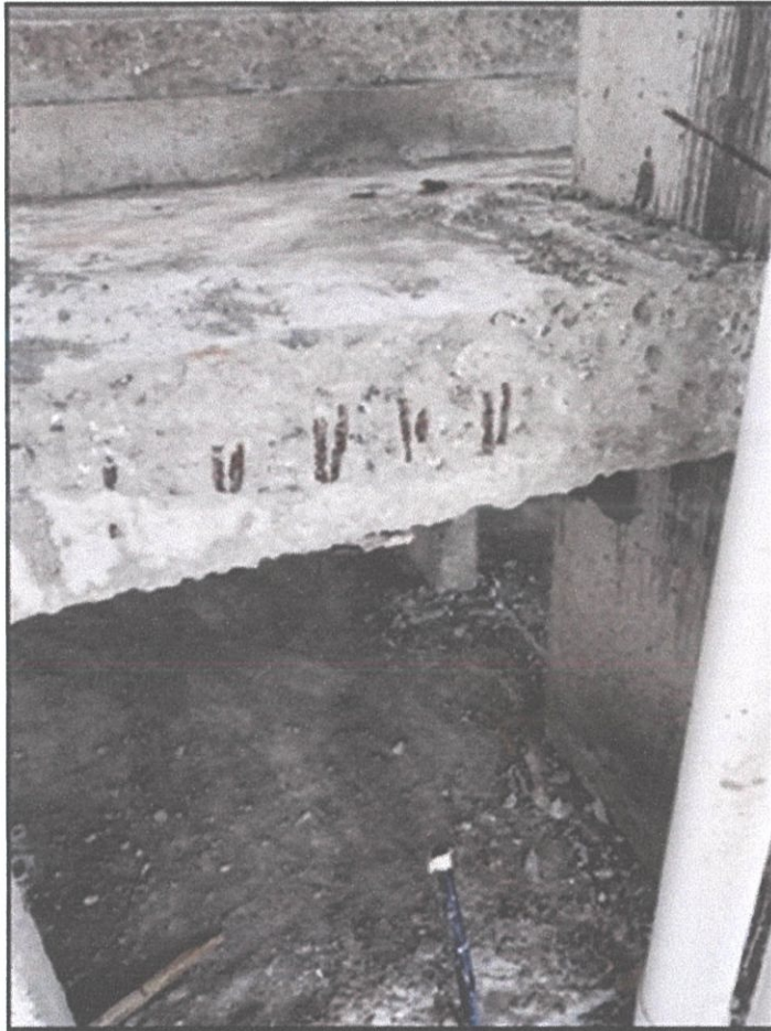
Figure 3.23 Steel bar visible out from structure
