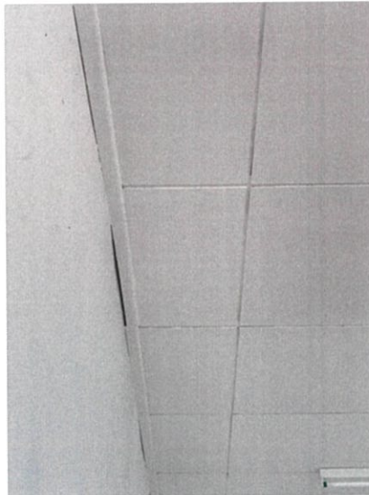
Figure 52.3.1: Gap between fixed ceiling and wall
