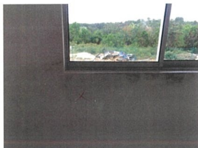
Figure 20.3.1: Dampness on wall.
