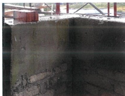
Figure 19.3.1: Dampness on plaster brickworks.
