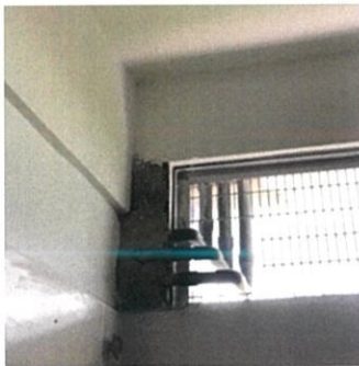
Figure 44.3.1: Improper installation of pipes in toilet
