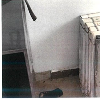
Figure 37.3.1: Improper arrangement of tiles skirting
