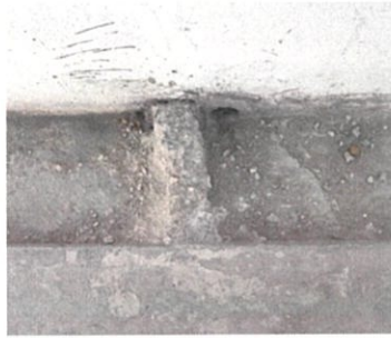
Figure 41.3.1: Excessive cement in scupper drain
