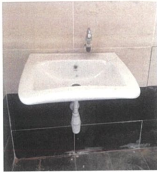
Figure 48.3.1: Non-alignment of tap pipe and sink
