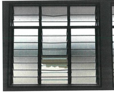
Figure 47.3.1: Window rods bend
