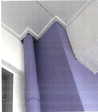
Figure 51.3.1: Gap between piping and column
