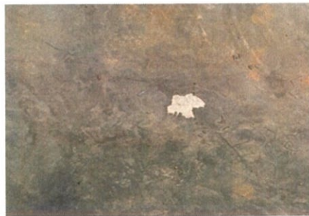
Figure 35.3.1: Delamination of concrete
