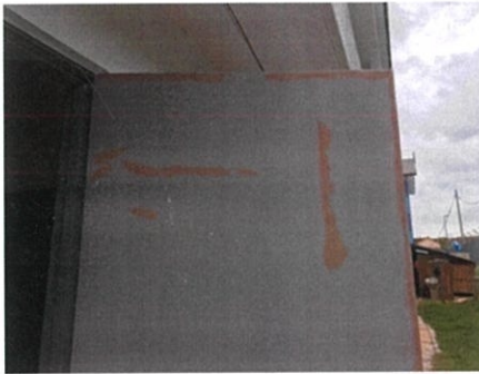
Figure 16.3.1: Improper painting on door panels.
