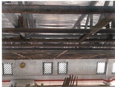
Figure 21.3.1: Timber panel of roofing structure decay
