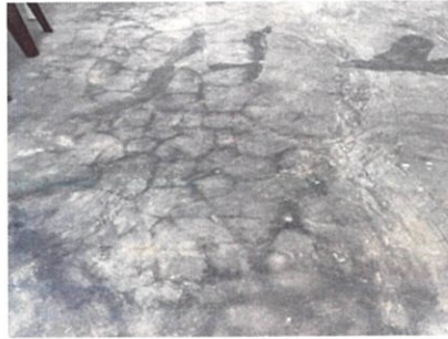
Figure 34.3.1: Crazeing on concrete floor
