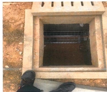
Figure 45.3.1: Wrong design of trash grill
