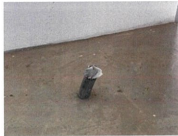
Figure 43.3.1: Exposed pipe on floor
