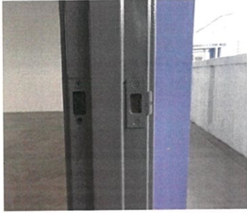
Figure 46.3.1: Improper installation of ironmongeries
