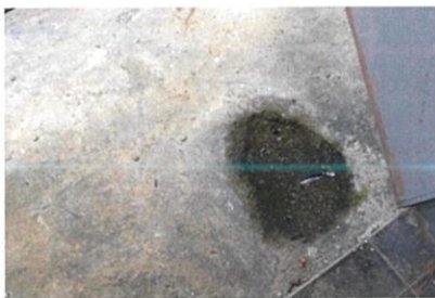
Figure 22.3.1: Mould on concrete
