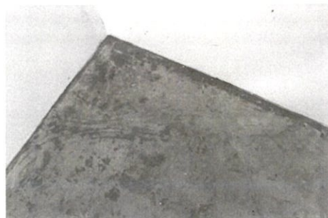
Figure 36.3.1: Dusting of concrete
