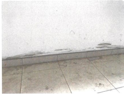
Figure 17.3.1: Stains on walls
