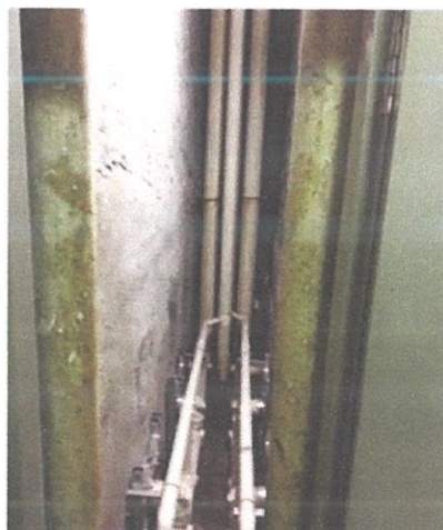
Photo 3. 3 Pipe leaking at level 3
