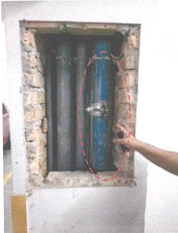
Photo 3.3. Leaking (blue) pipe
