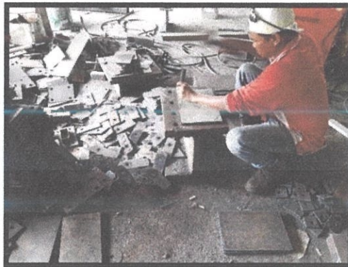
Figure 3. 10: Labor was marking the plate using a sledgehammer and a center punch.
