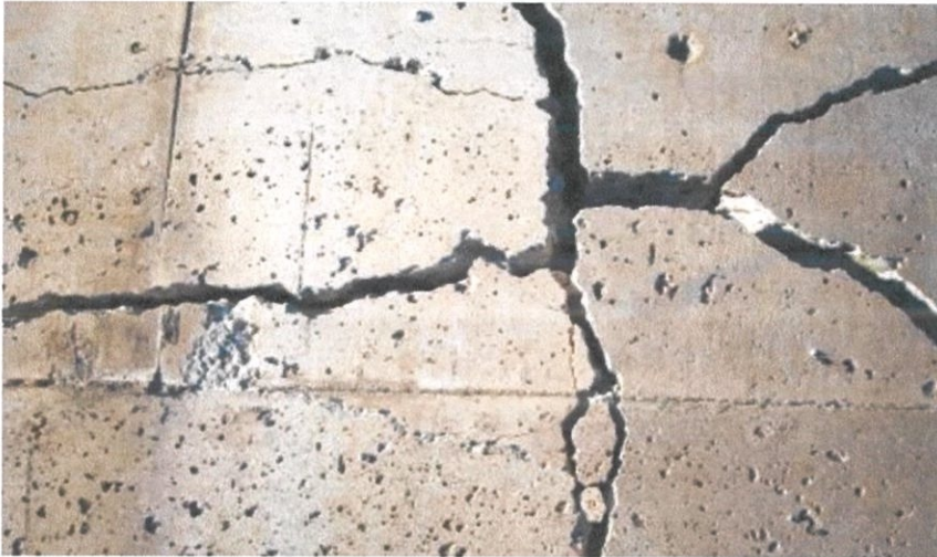
Figure 3.12 cracking in concrete
