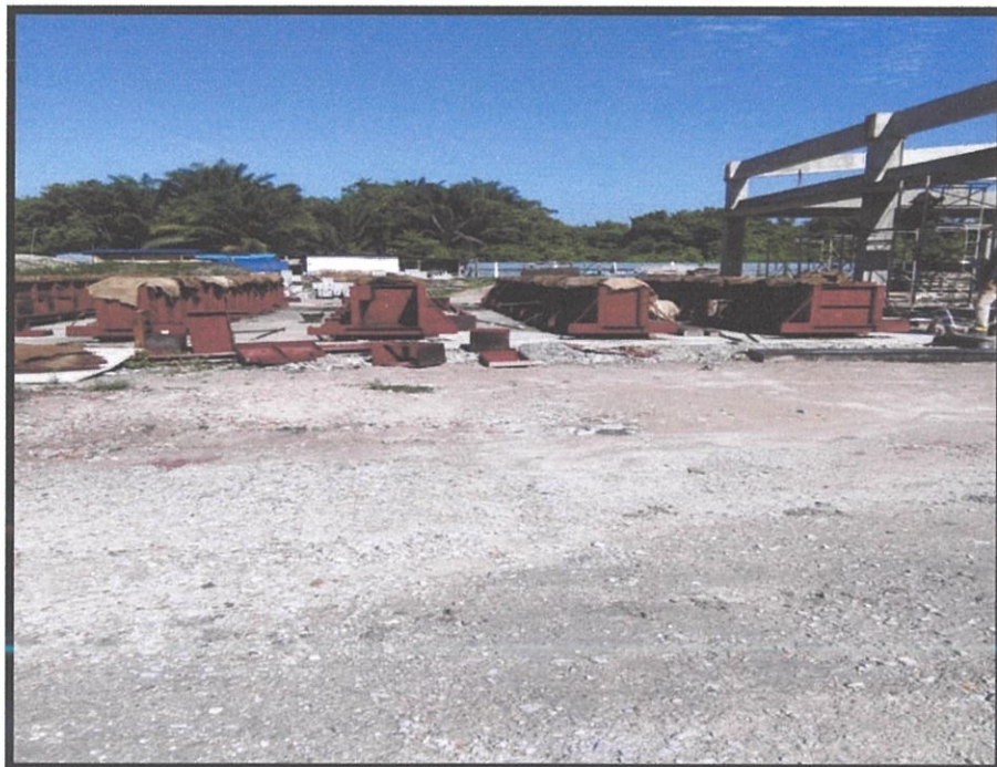
Figure 3.10: The precast elements in steel moulds are cured and enclosed with gunny sacks
