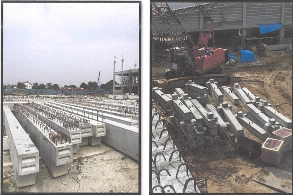
Figure 3.13: The precast elements are placed and stored at a designated space on site
