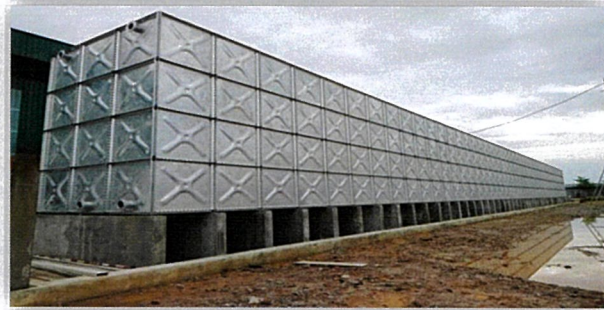
Figure 1 : Hot Dipped Galvanised Pressed Steel Water Tank
