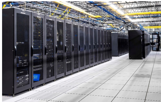
Figure 3: Example of data centre that use in CSF Advisers Sdn Bhd
