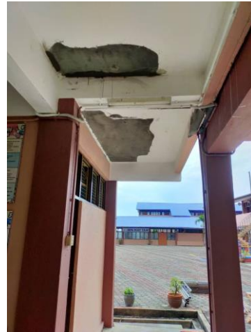
Figure 21: Damaged of Ceiling
