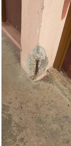
Figure 18: Damaged at The Column
