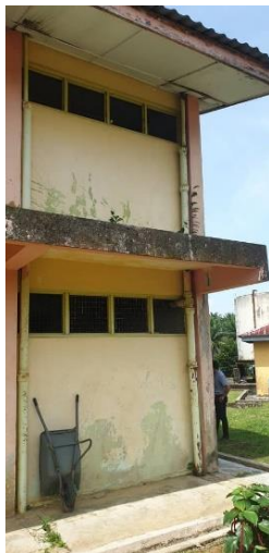
Figure 18: The Color of the Building Has Faded
