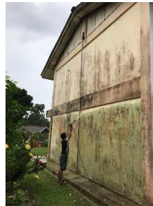
Figure 35: Wash out of Old Paint at The Exterior Wall
