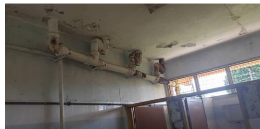
Figure 23: Leaks On UPVC Pipes
