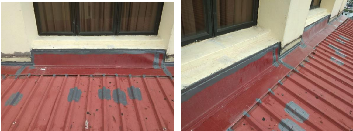
Figure 16: The flushing roof that has been installed and putted silicone to prevent leakage
