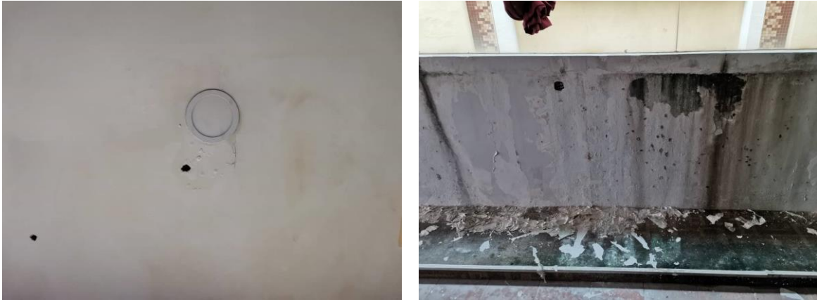
Figure 17: Damaged ceilings and walls
