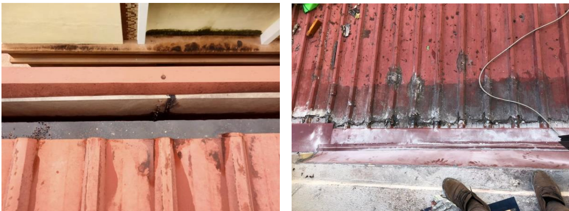
Figure 6: The gutter that full of garbage and the roof that has damaged
