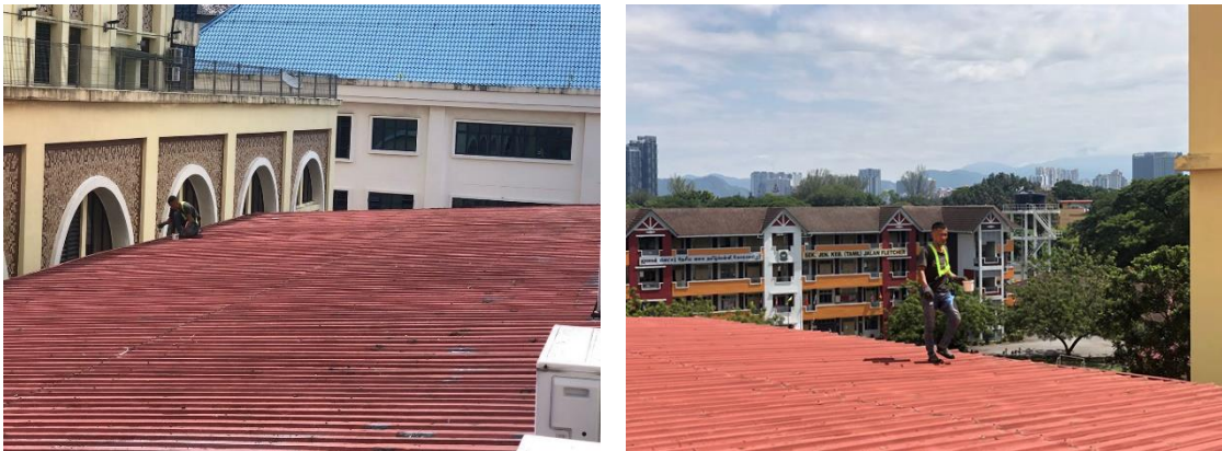
Figure 12: The workers are attaching waterproofing tape and silicone to the damaged roof
