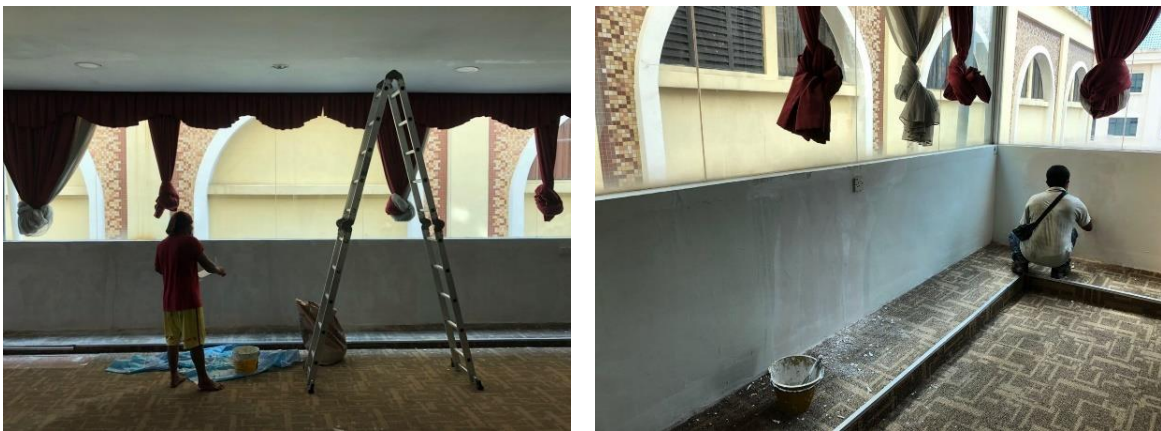
Figure 18: The work of putting sealers on the ceiling and the work of painting the walls
