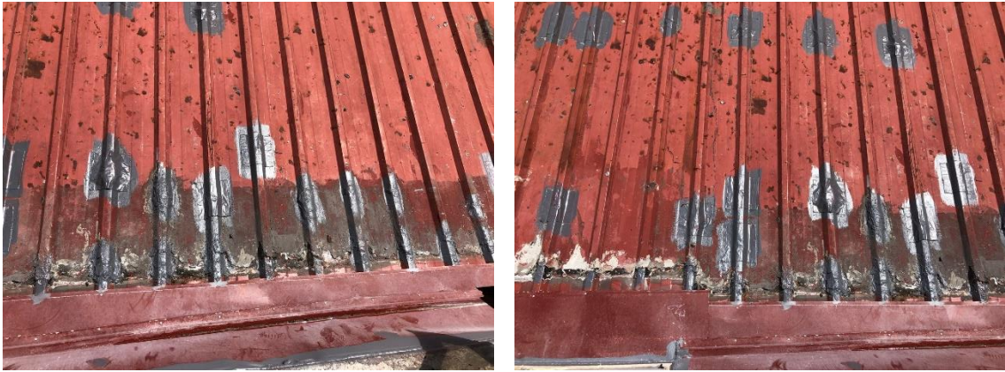
Figure 11: Damaged roof that was attached with waterproofing tape and silicone
