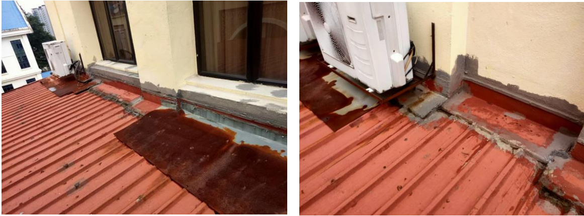
Figure 5: Flushing roof that already rusted
