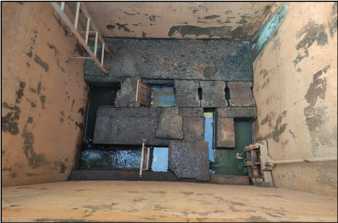
Figure 14: Primary Screen Chamber
