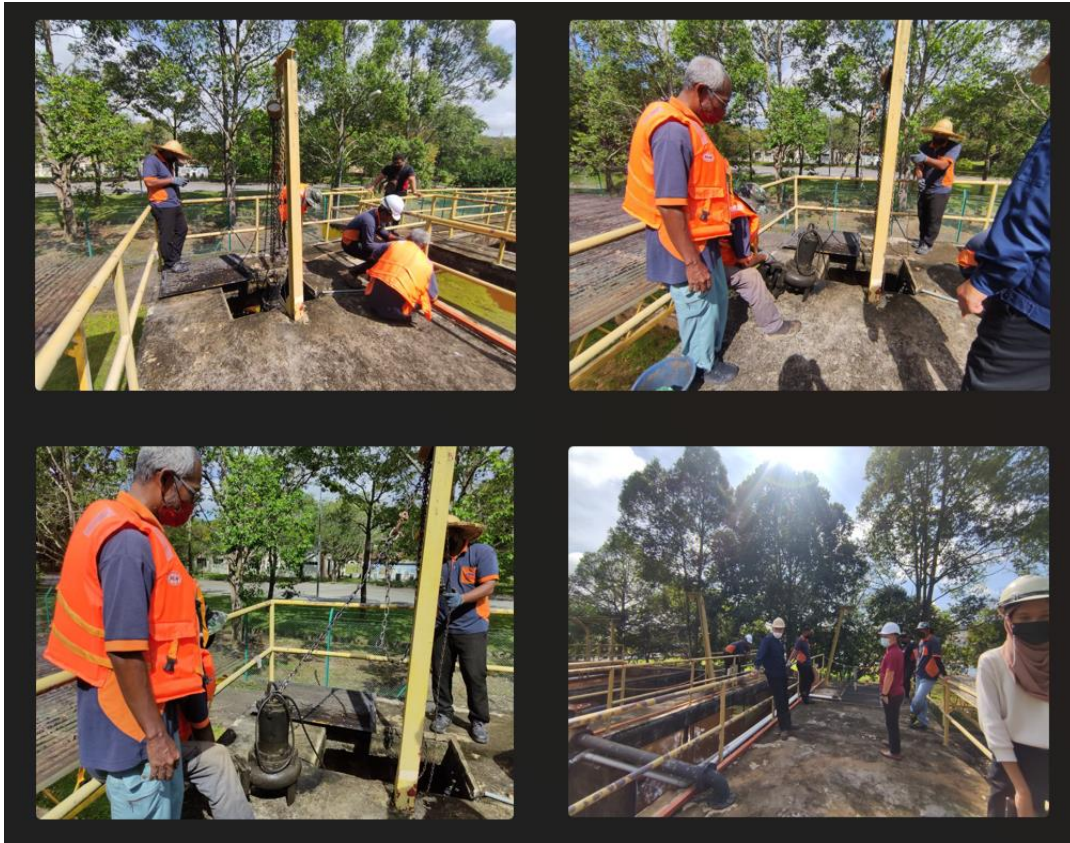
Figure 25: Left Ras Pump at Holding Tank
