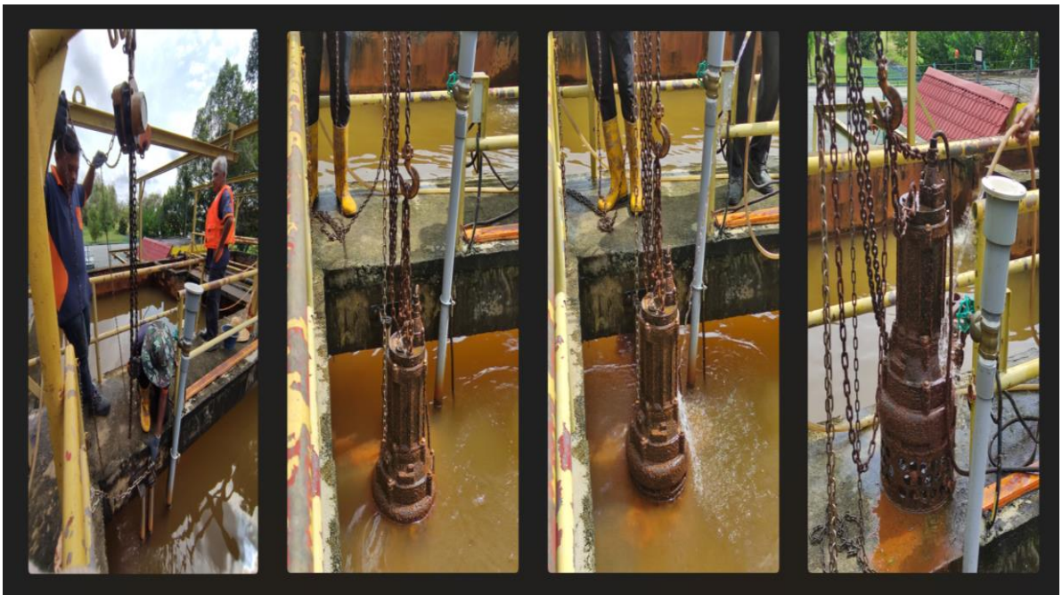
Figure 22: Ejector Pumps at Left Aeration Tank
