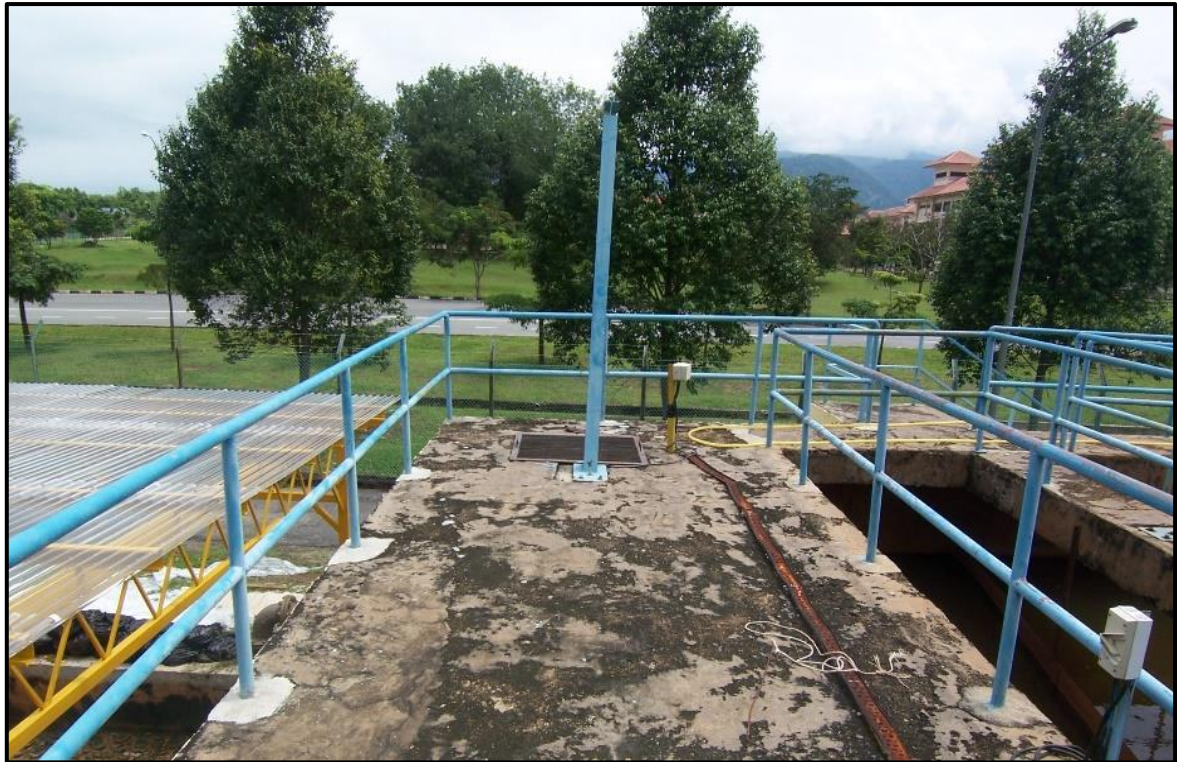
Figure 18: Sludge Holding Tank
