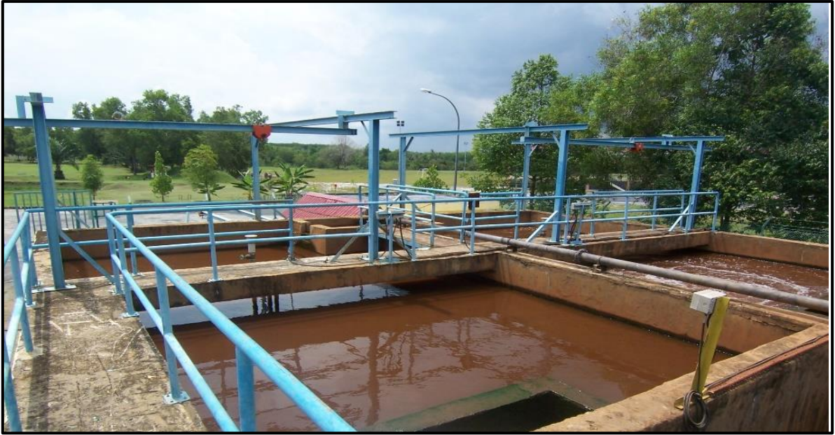
Figure 21: Aeration Tank At STP 1
