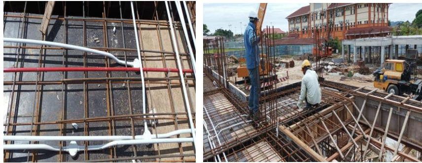
Figure 3. 43: The situation when the electrical workers doing their work to apply the PVC pipe in the slab area
