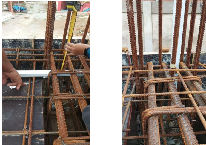
Figure 3. 44: The situation for setting out and marking for the level of concrete
