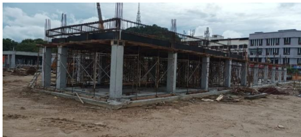
Figure 3. 37: The view in the construction site when the reinforcement bar for beam finish
