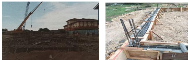
Figure 3. 28: The condition of the formwork after the completion of the concrete activity
