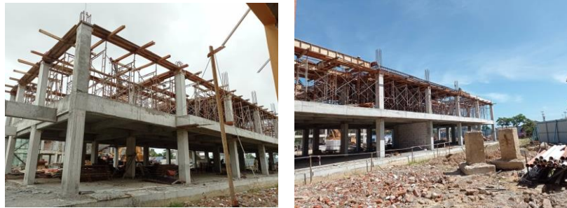
Figure 3. 36: The view in the construction site during the beam and slab process
