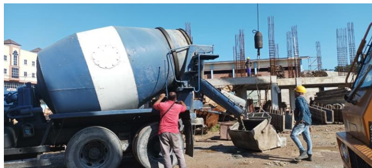
Figure 3. 47: A view when the worker pours the concrete into a concrete bucket
