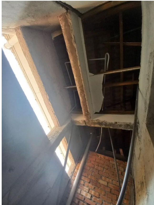
Figure 3.6: View at the site that the work should have been done last year, 2021 but do not have any progress until year 2022.
