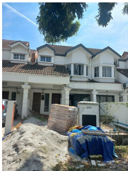
Figure 3.2: View of the site that had no worker to continue the house renovation.
