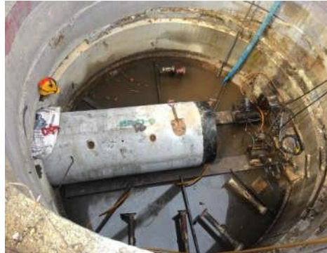
Figure 3.7: Process of lowering the first length of reinforced concrete pipe Source: PDP's document, 2021
