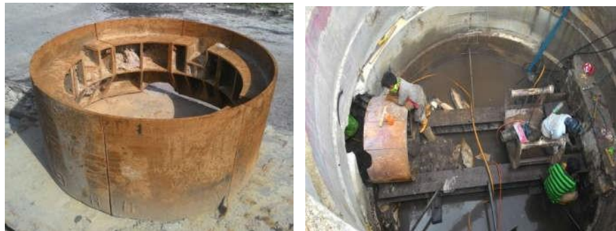
Figure 3.6: Cutter head of the pipe jacking and the process of position it into place Source: PDP's document, 2021
