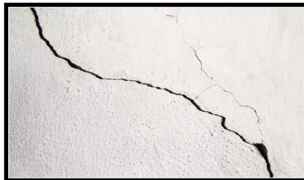
Figure 6: Cracking of wall (Alisa Ivanova, 2016)
