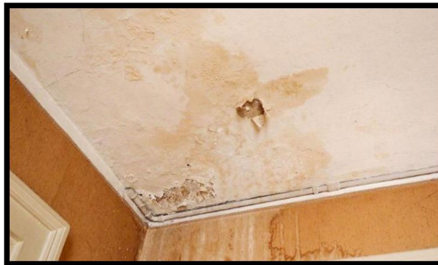
Figure 9: Dampness (Nurul Nadia Omar Bakri, 2014)
