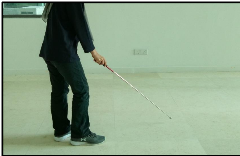
Figure 30: Process of identifying hollowness of floor tiles by using a tapping rod
