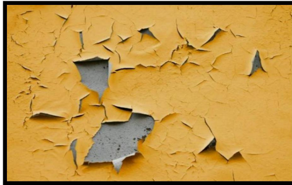
Figure 5: Peeling of paint (Bob Vila, 2015)
