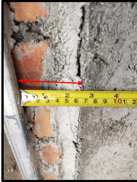
Figure 3. 19 The gap between column and door frame
