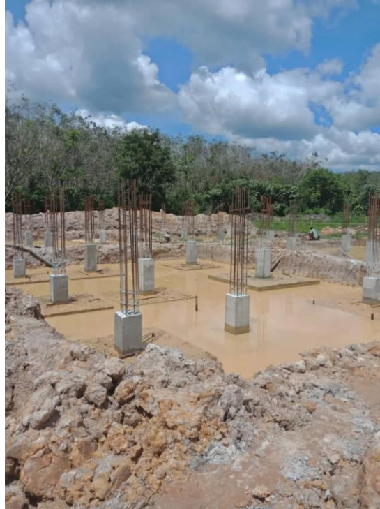
Figure 3.17: Water stagnate during construction
