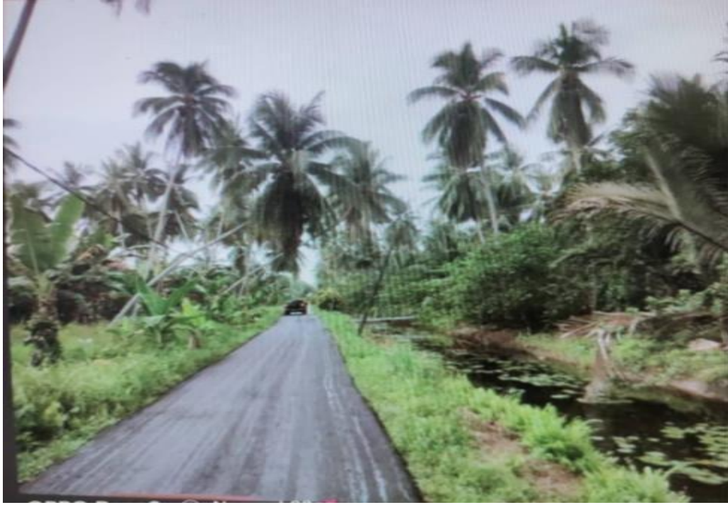
Photo 2.9 Road mentainance at “Jalan Rizab Tengah from Kg Tebuk to Kg Sg Batang
