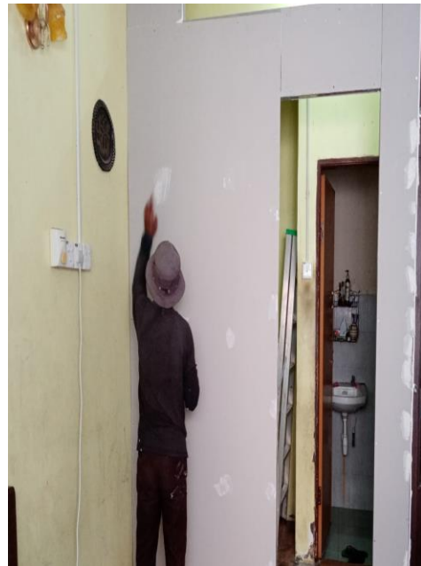
Figure 6: The employee filled the gap has been patched fiber tape with a mixture of new bonding cornice
