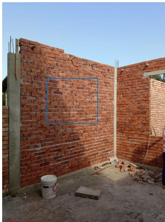
Figure 3.23: The wall where there should be a double leaf window
