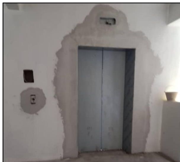
Figure 7: Single-speed center opening system door at Sungai Pinang Apartment
