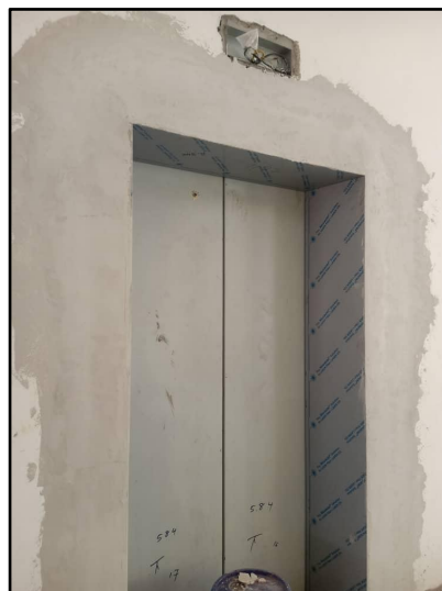
Figure 12: Traction Geared Elevator door panel
