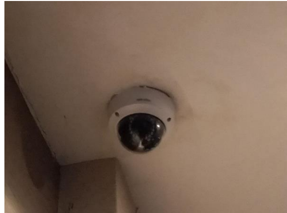
Figure 3.2: CCTV in Grand Ballroom hall
