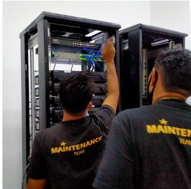
Figure 4.2: Maintenance staffs do monthly survey at control room
