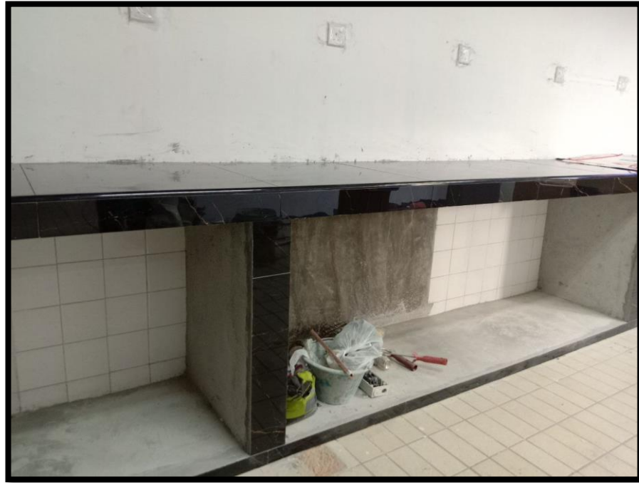
Figure 7: Concrete bench without wooden cabinet
