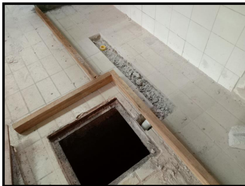
Figure 5: The position of the waste sum/manhole
