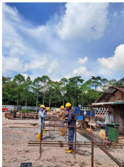
Image 2.1: Labors are not wearing a proper safety boot.
