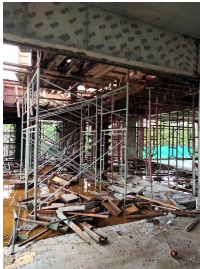
Image 2.0 : Improper stored of plywood that have been used.
