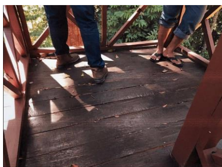
Figure 3.11: Rotten Floor Hostel
