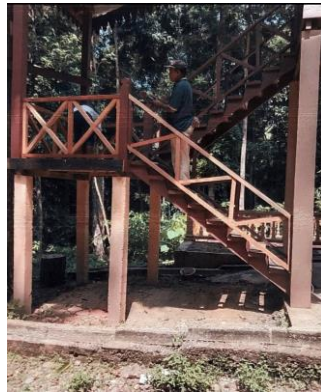
Figure 4.22: Railing Before Maintenance
