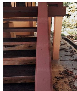
Figure 3.12: Rotten Railing Fence
