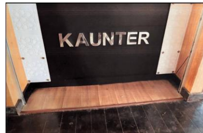
Figure 4.17: Signage "KAUNTER" After Maintenance
