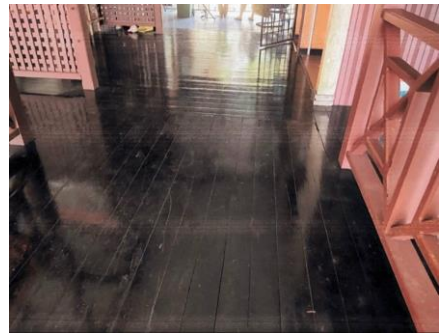
Figure 3.6: Rotten Floor Jetty
