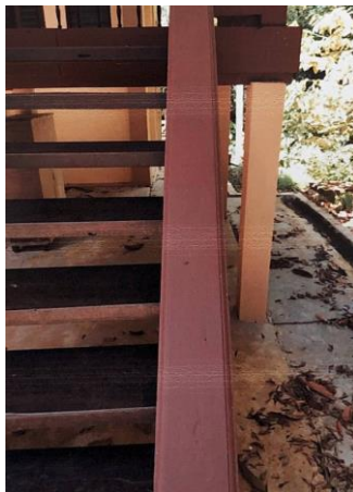
Figure 4.20: Railing Before Maintenance
