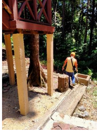
Figure 4.28: Sump During Maintenance
