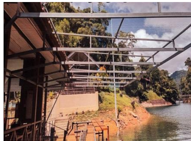
Figure 4.8: Awning Before Maintenance
