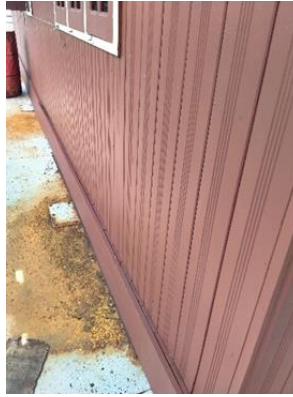
Figure 4.11: Floating Before Maintenance
