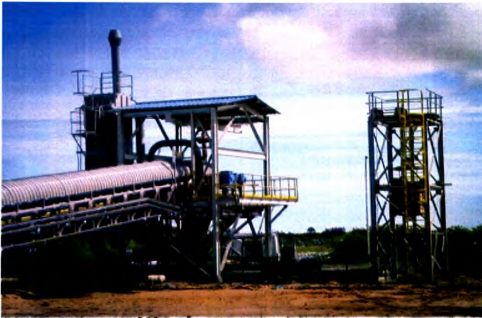
Dust Collector and End Tower for coal Conveyer System ( Mukah Coal-Fire Power Plant )
