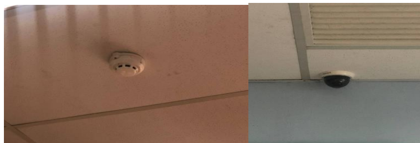
Figure 22: Smoke Detector and CCTV
