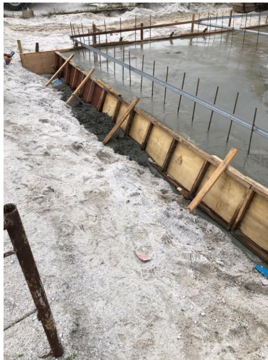
Figure 3.19: Problem concrete overflow from formwork
