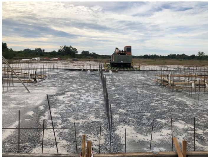
Figure 3.18: Problem Concrete in Raining
