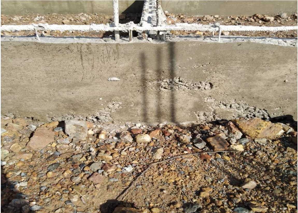
Figure 14.0: The honeycombing in the concrete formed and spotted after the formworks were opened
