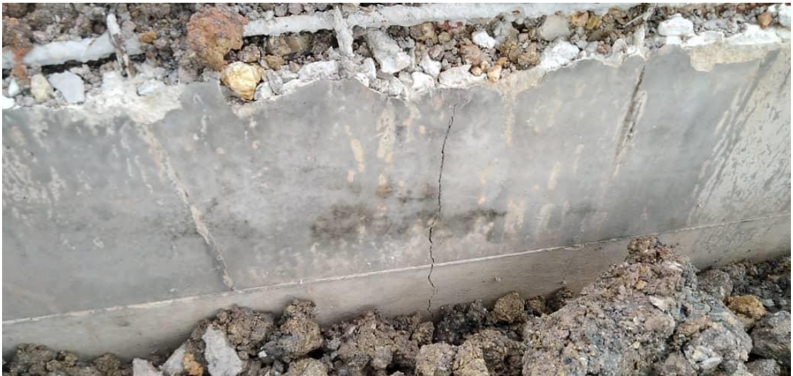
Figure 13.0: The cracks that been spotted during the inspection
