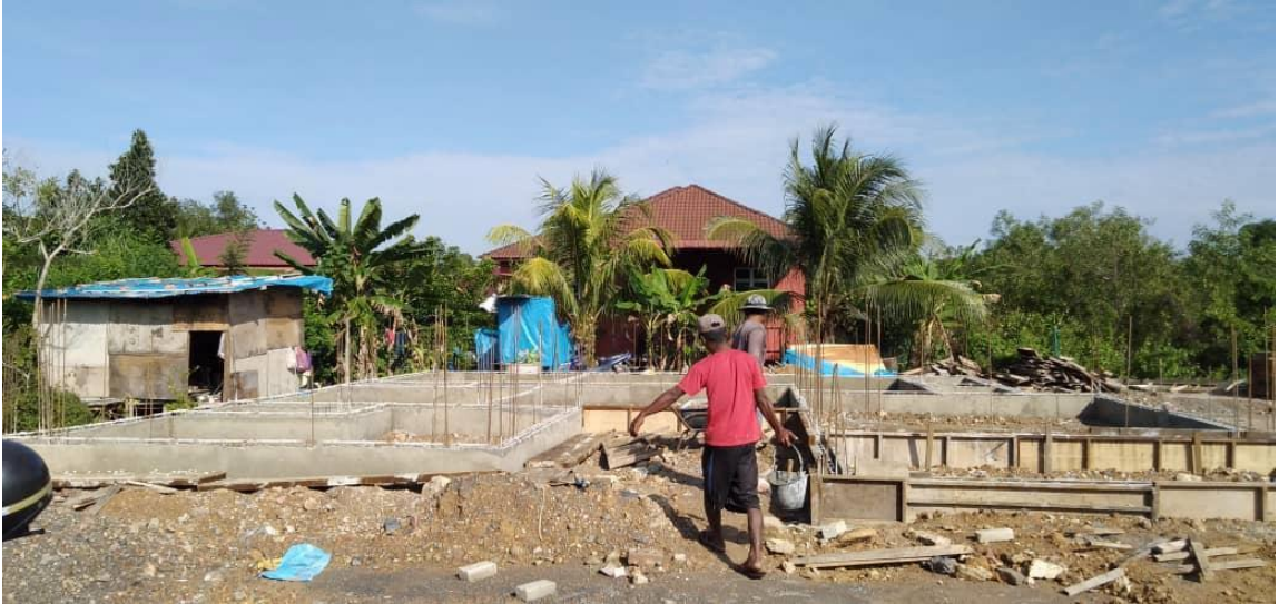
Figure 15.0: The worker batched the epoxy of cement-based to patch at the crack and honeycombing.
