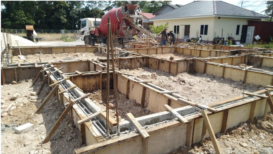
Figure 9.0: The concreting process of the reinforced beam using the ready mix concrete carried by a concrete mixer truck.
