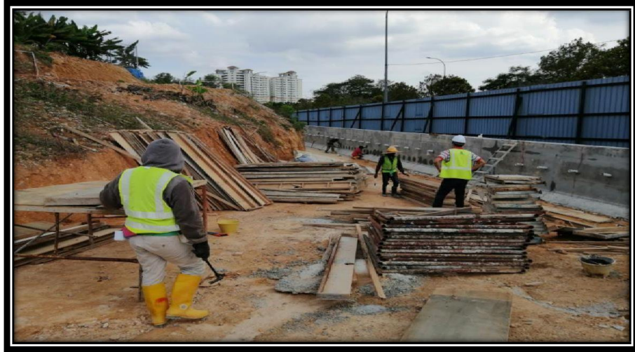
Figure 7: Shows the worker does not wear safety helmet and boots at site
