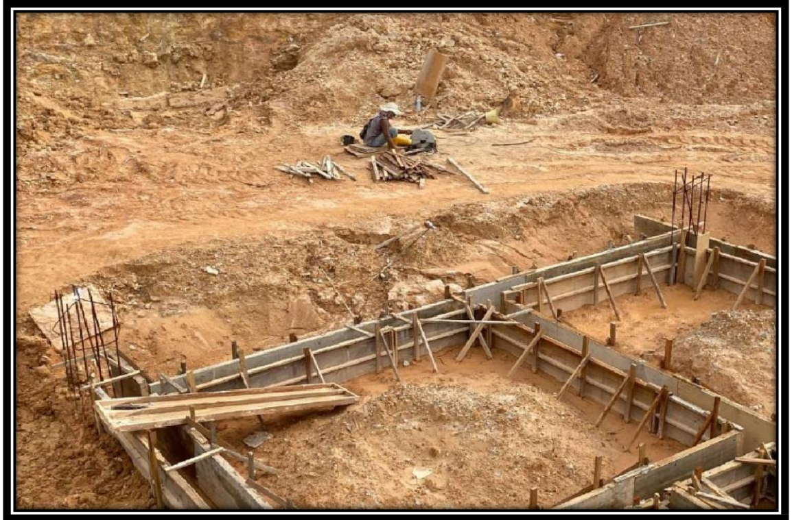
appendices 3:Shows the worker cutting the hardwood for making formwork for work lower ground
