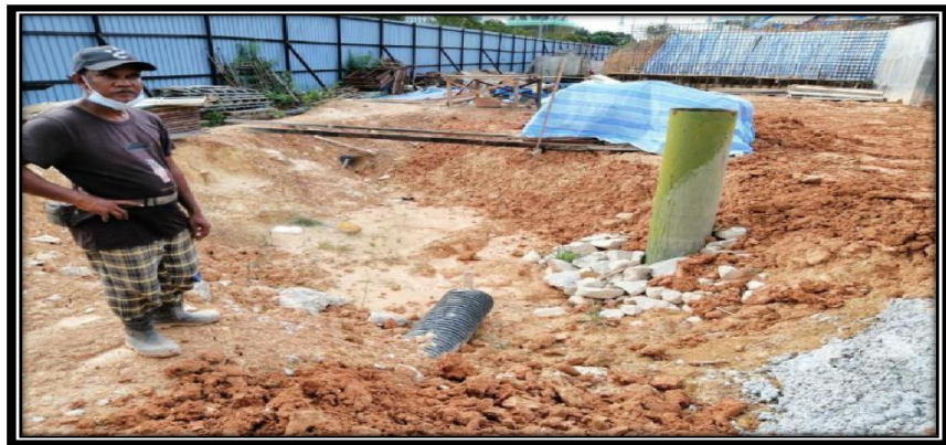
Figure 6: Shows poor safety compliance at site
