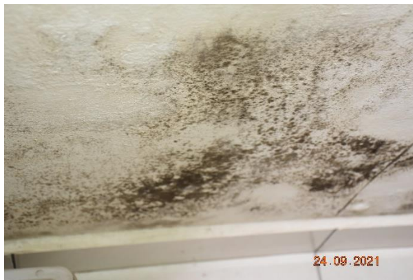
Figure 3.6: Water stain mark on wall.
