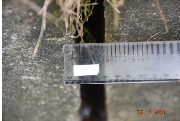
Figure 3.3: Crack on road drain
