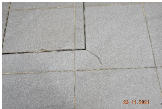
Figure 3.2: Crack on floor tiles
