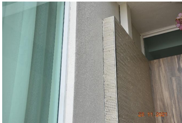
Figure 3.5: Separation gap on wall tiles.
