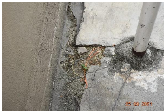
Figure 3.4: Chipped off cement screed.
