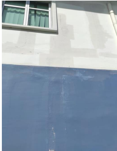
Figure 3.10: Defects detected behind Administer Building
