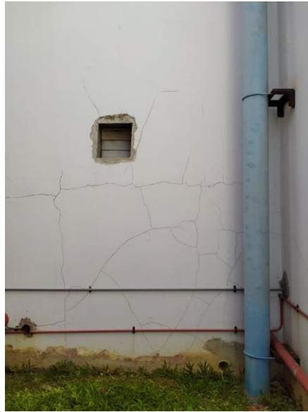
Figure 3.8: Defects behind Chiller Plant building in UiTM Jasin
