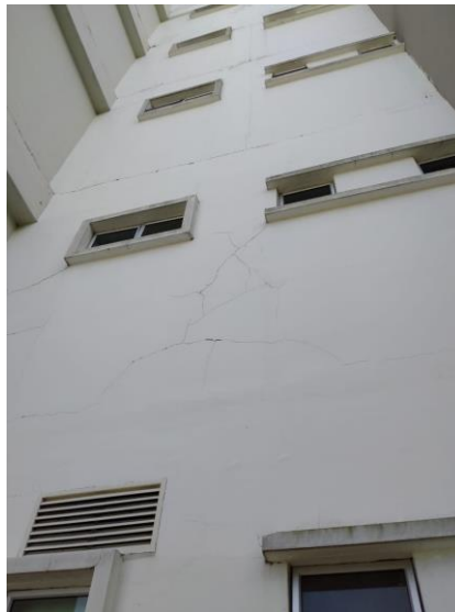
Figure 3.9: Defects behind 'Blok Kuliah' in UiTM Jasin
